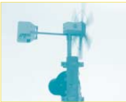
▲ This remote radio repeater in Kananaskis, Alberta uses solar energy to produce electricity in addition to wind. (Photo courtesy of Norwester Energy Systems Ltd.)
